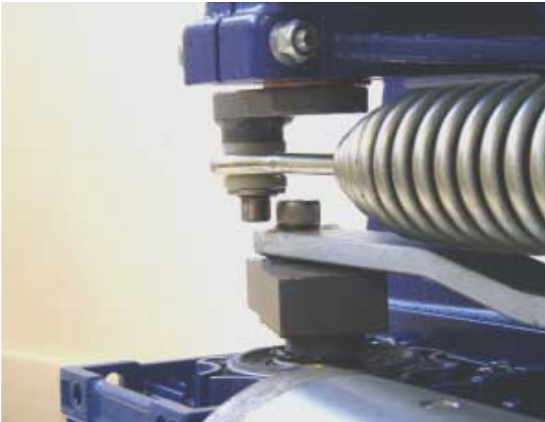
PHOTO, GAP BETWEEN SHAFT AND ALLEN BOLT
